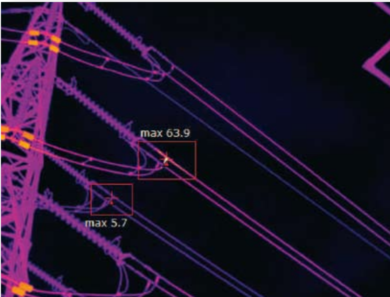
Image taken with 640x480 pixel resolution and <45mK thermal sensitivity. Notice how the hot spot now is clearly visible and that the increased number of pixels will result in an even more accurate temperature reading in the hot spot. It is now clear that there is a problem in the power line.
